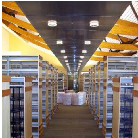
A perforated metal soffit delineates the main circulation through the book stacks.
